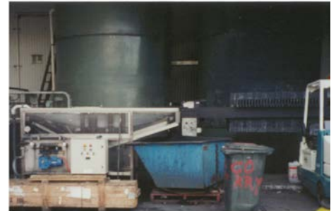
General arrangement of V-FOLD™ before removal of “plate and frame” filter.
